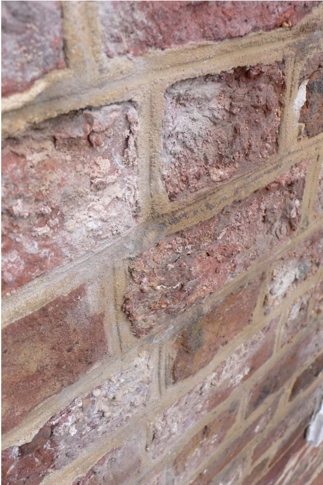
Again salt at the surface and brick faces beginning to exfoliate behind the 1950s portland pointing.
